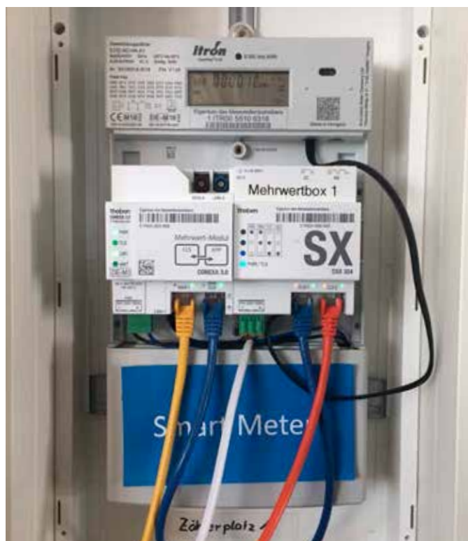
Fig. 2 - Smart Meter Infrastructure providing secure bidirectional communication with decentralized energy systems. The Smart Meter is shown in the background. The Smart Meter Gateway (secure router) is the Connexa 3.0 CX component on the left side. The SX-module on the right side hosts the secure communication with the solar inverter, storage or e-charging wallbox (Photo: © THU, Theben AG).
