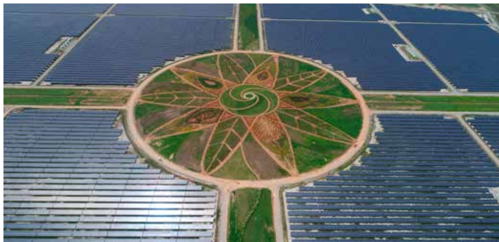
Fig. 1 - 98 MW PV system at Haenam-gun, Jeollanam-do, Korea.
