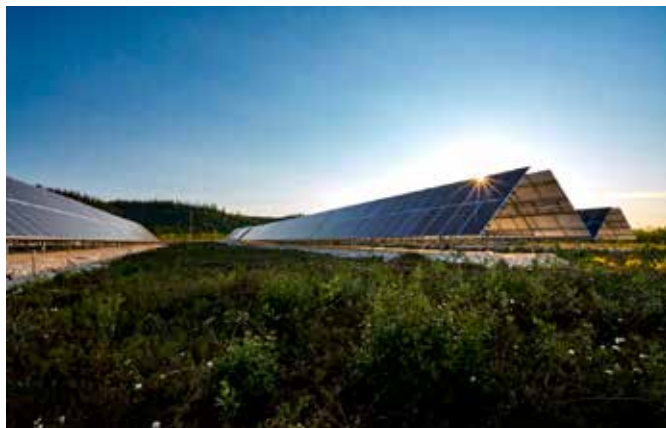
Fig. 1 - The Old Crow Solar Project, a 940 kW system installed by the Vuntut Gwitchin Government in Old Crow, Yukon, 128 km north of the Arctic Circle (Photo: Solvest Inc.). 3
