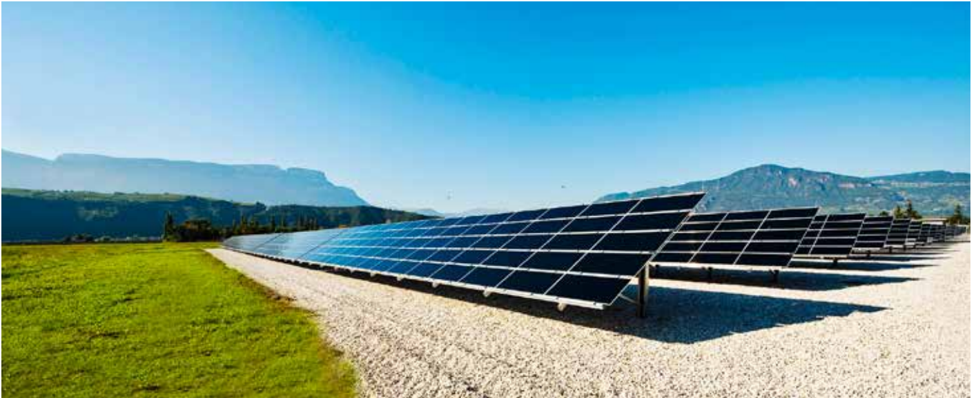
Fig. 1 - A multi-technology photovoltaic test facility for the detailed performance evaluation of different module technologies and mounting systems was set up by EURAC research in cooperation with Airport of Bolzano Dolomiti (ABD). It is operating since 2010 (Photo: EURAC /Othmar Seehauser).
