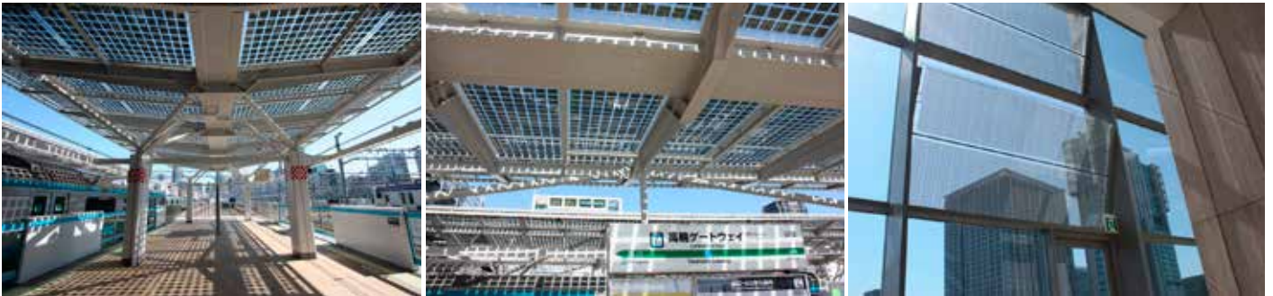
Fig. 1 - Roof and Window Glass-integrated PV System at Station Platform (Takanawa Gateway Station PV System) (Minato Ward, Tokyo). Power generation capacity: 43.8 kW (roof of platform), 1.1 kW (window glass). PV modules: Bifacial single-crystalline silicon PV modules (SUNJOULE® glass-integrated PV modules by AGC).
