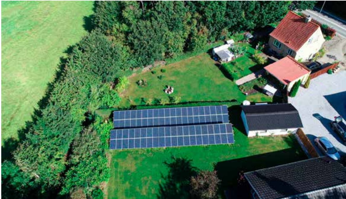
Fig. 2 - Vester Skerninge, Fyn. Privately owned with 20 kWp PV plant with a 16 kWh lithium battery (Photo: KlimaEnergi A/S).
