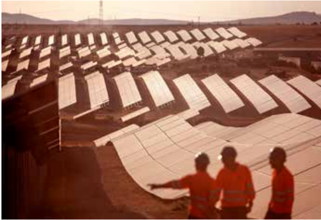
Fig. 7a - Construction of “Nuñez de Balboa” PV plant (500 MW in Badajoz, Spain) by the Spanish utility IBERDROLA.
