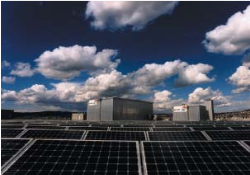
◀ Figure 1.2: Flat roof integrated photovoltaic installation with solar power of 270 kWp feeding the grid in Zurich. Copyright: Zollfreilager, Switzerland.
