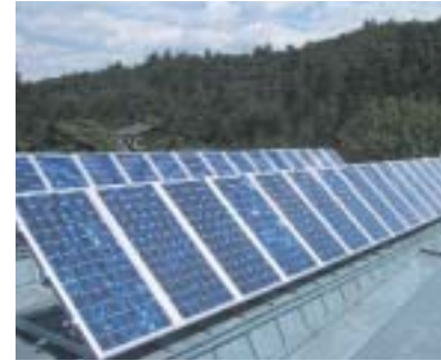
▲ Figure 7.6: Pilot Project “Institute Frankenberg”. Location: City of Bolzano (Italy). Installed capacity: Grid-connected 3.1 kWp. Financing: Italian Ministry of Industry (MICA) and autonomous Province of Bolzano. Source: courtesy of Gechelin Group Sistemi Fotovoltaici, Italy.
