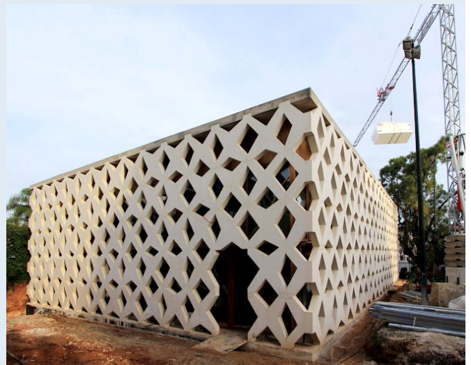
New chancellery building in Algiers, Algeria. The white concrete facade is earthquake-resistant and protects the building shell against sunlight.
