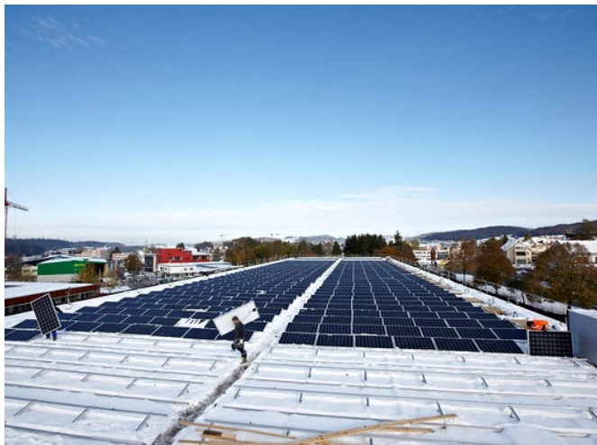
Installation of the photovoltaic system on the roof of the collections centre of the Swiss National Museum in Affoltern. The output data may be monitored via the following web site: http://gemperle.solarlog-web.ch/11861.html .
