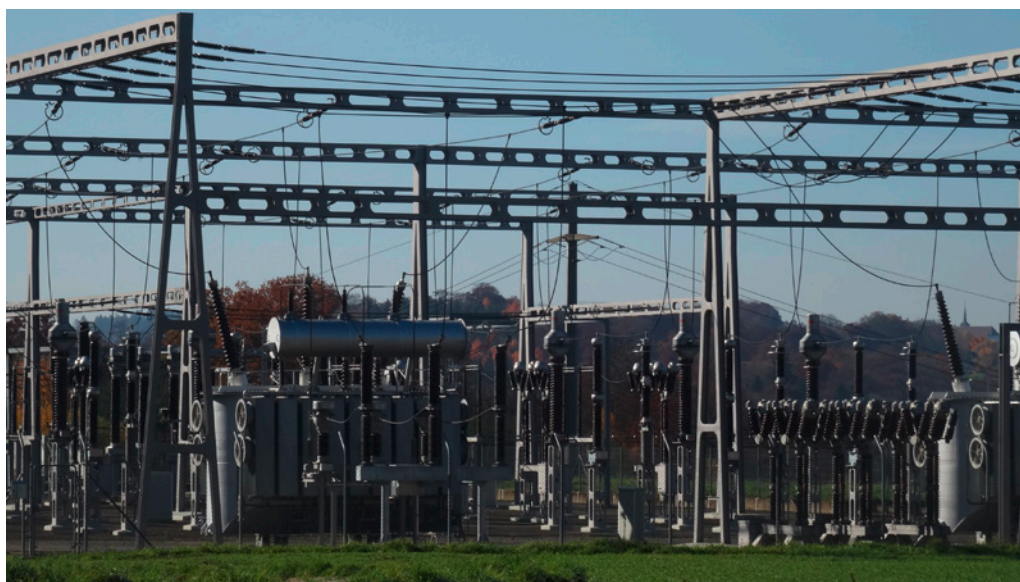
Transformatorstation in Chésalles (Marly). Quelle: Marcel Gutschner
