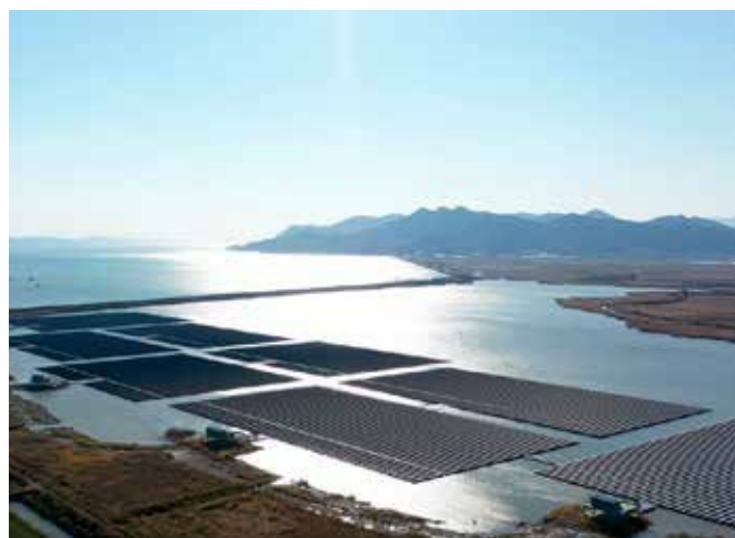
Fig. 3 – 25 MW Floating PV system at Goheung-gun, Jeollanam-do, Korea.
